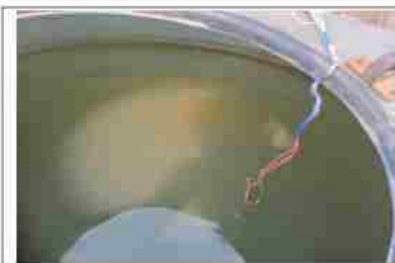
Sensor inside the overhead tank
