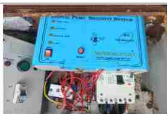
Control Circuit in the pump house
